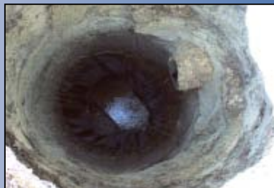
Precast manhole experiencing high deterioration and corrosion with exposed reinforced and structural fatigue
